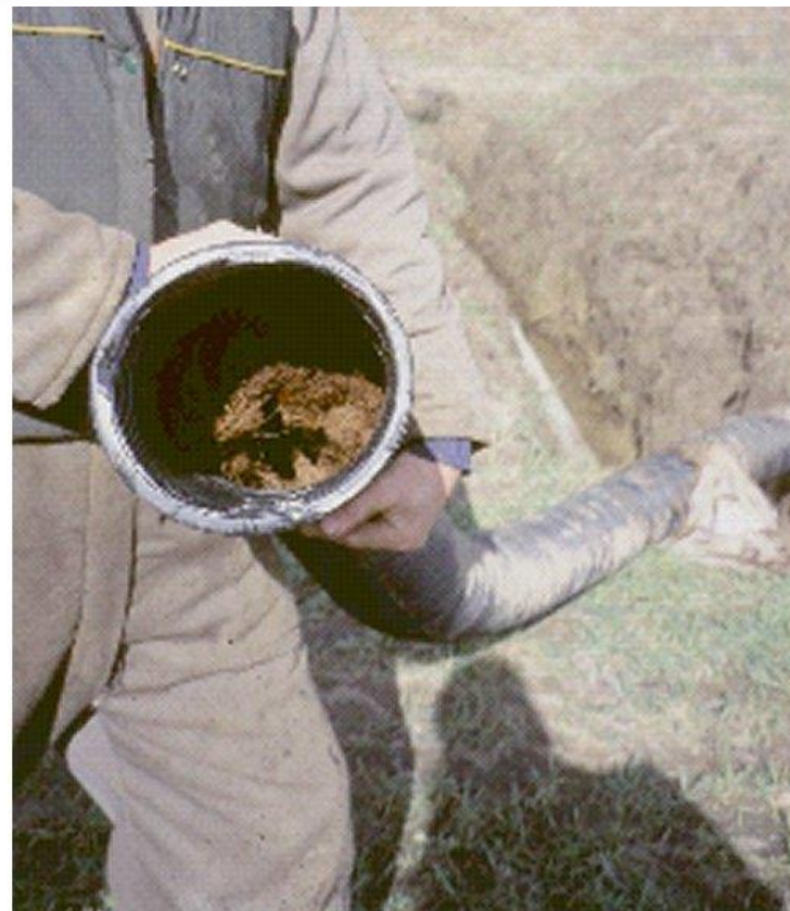
Figure 2. A lengthy section of 10 inch mainline is plugged solid with roots. The roots originated from a large willow tree located more than 50 feet away from the buried drain.
